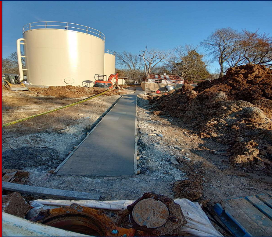
New 130,000 Gallon Storage Tanks in Preston Shores
